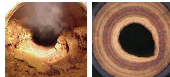
Depending on the composition of the distribution piping, a variety of substances including copper and iron can be dissolved in and contaminate the water.
